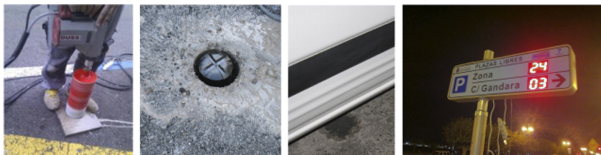
Figure 7.5 Examples of parking sensors installation and guidance panels
